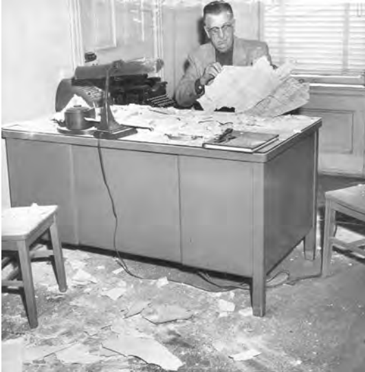
January 1954 Sheriff Ed Kiene inspects plaster that fell from the ceiling at the County Jail. Topeka Daily Capital - Staff
